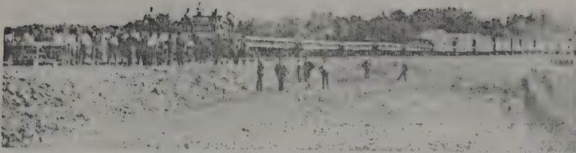
This picture, also taken by W. R. Long, was taken the day construction from the north reached Williamsburg. Note the ties and sections of track on the flat cars for continuing the road on south. The scene is at the north edge of town probably where the track crosses Old Man's Creek.
